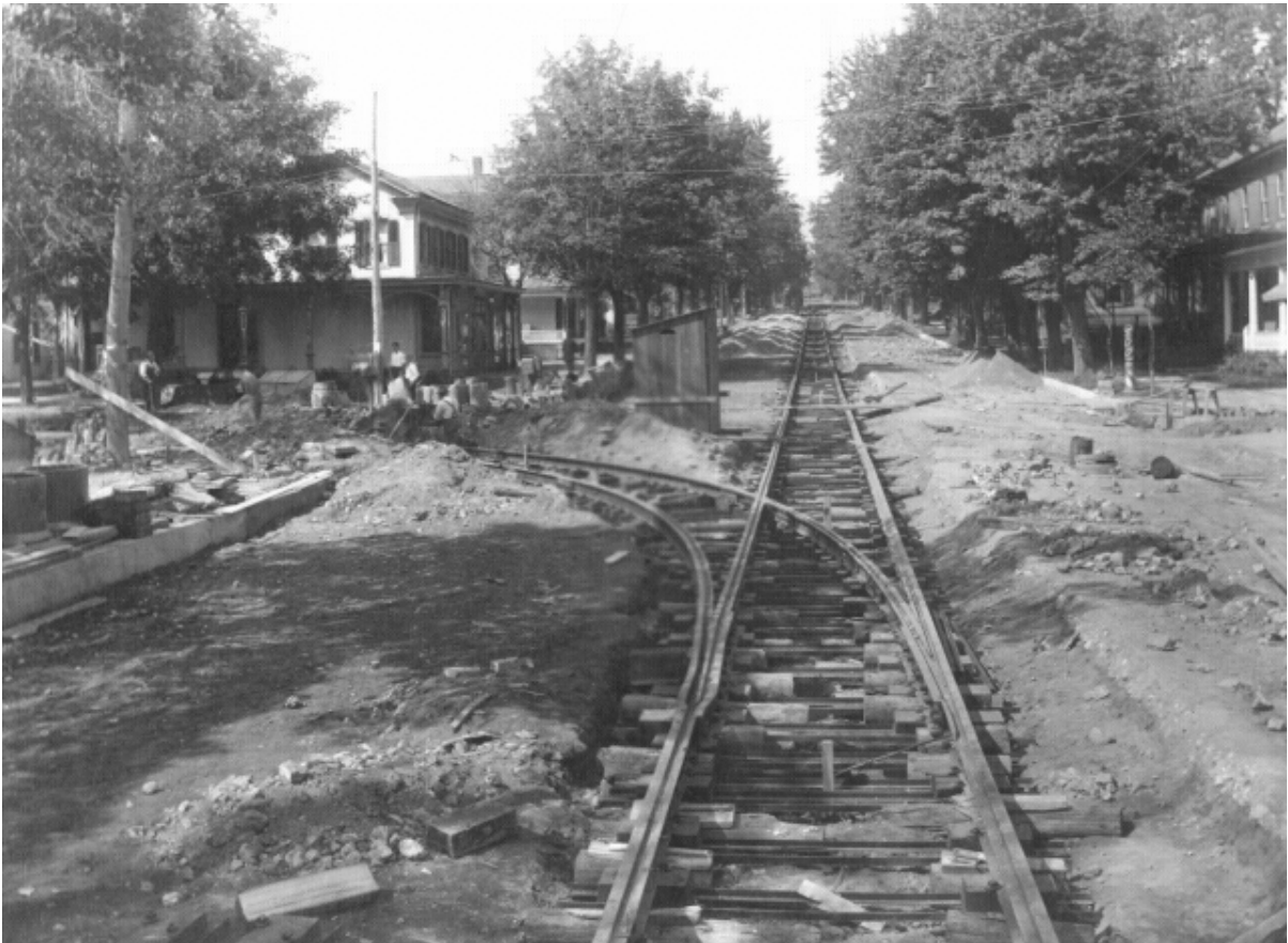
Construction of the Columbia & Montour Electric Railway Line at Fifth and East Streets
