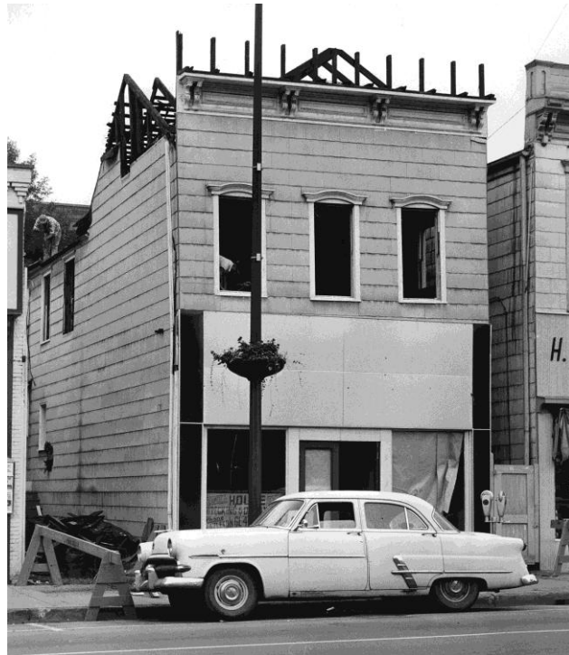
The longtime location of E. F. Row’s barber shop being dismantled, July 15, 1959
