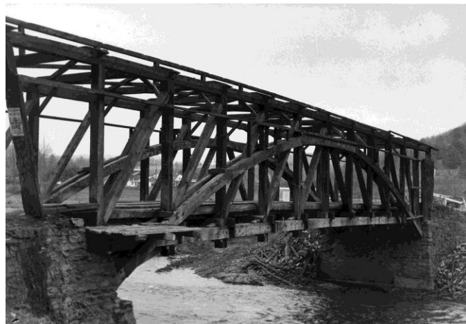
#130 Superstructure of a covered bridge at Forks showing the Burr arches (CCHGS 11-0086)
